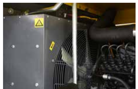
Enhanced cooling system for 50°C high ambient temperatures.
